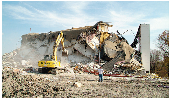
LAST REMNANTS of the Noah’s Ark Motor Inn comes down to make room for the Streets of St. Charles project that will get underway this Spring. Demolition work was by Premier Demolition, Inc.
